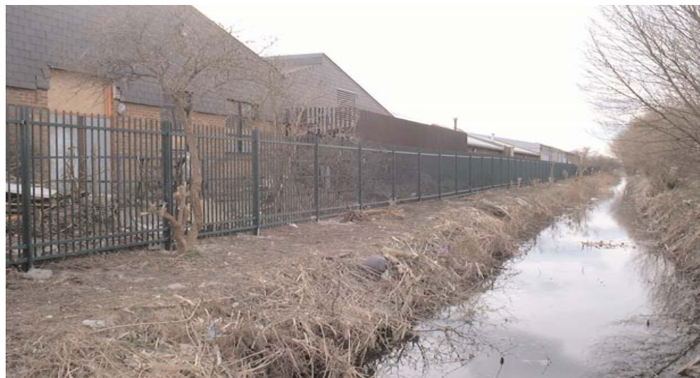
New fencing at River Road Industrial Estate, part of the Industrial Estates Revitalisation Programme
